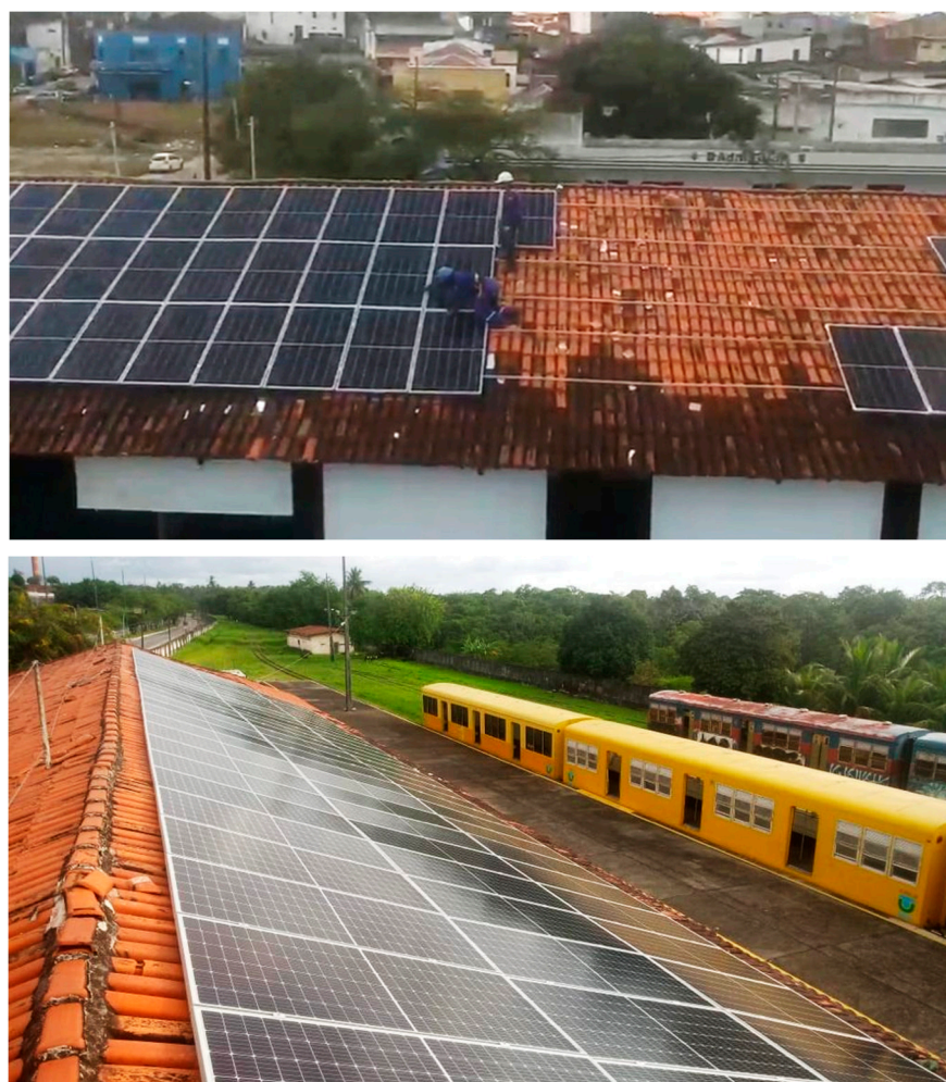
Figure 2. Photovoltaic systems from Joao Pessoa office during (top) and after (down) installation.
