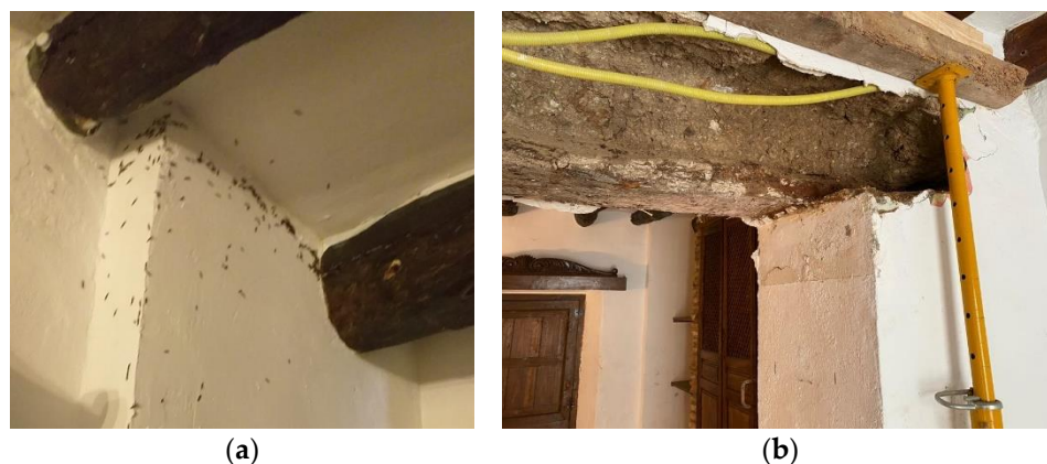
Figure 1. (a) Termite attack detected in a private home in Albuñuelas (Granada, Spain); (b) Intervention to replace damaged beams.
