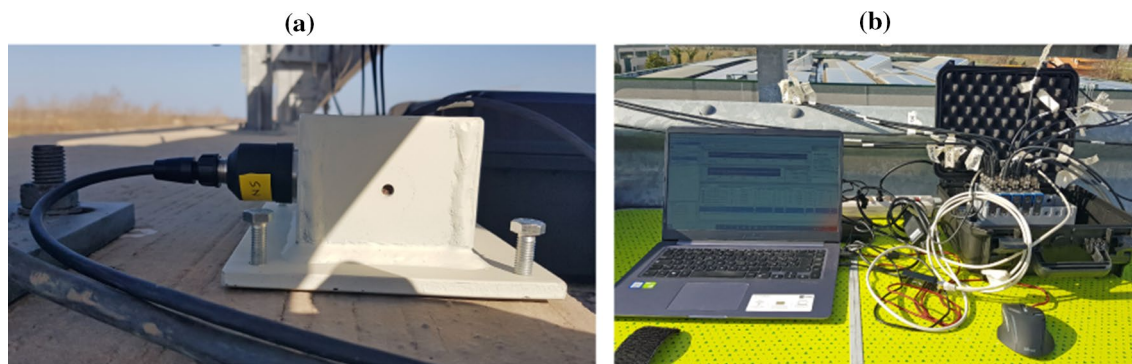
Fig. 5 Photographies of an accelerometer fixed to a steel support (a) and the DAQ (b)
