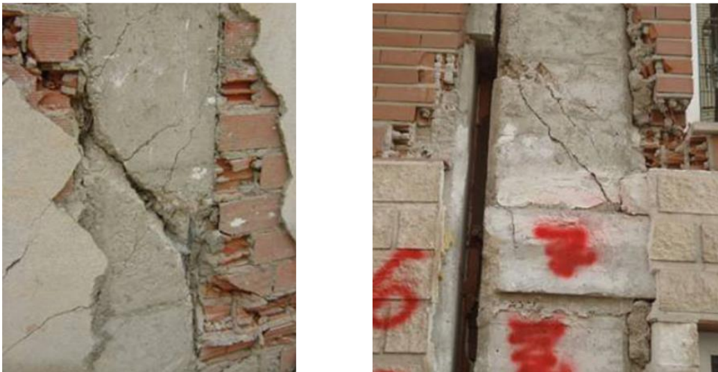
Figure 1. Shear deformation of columns during the Lorca earthquake (2011), adapted from [8].
