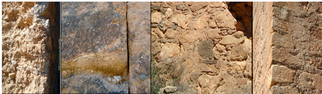
Figure 7. Materials used in the construction of Lojuela Castle (without scale). Source: PREFORTI project.
