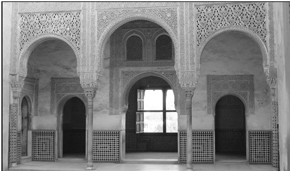
Figure 33. Cuarto Dorado portico showing the complete replacement of alicatado work on both the dadoes and the engaged columns. Photograph by Abelardo Alonso Gallardo, 19 November 1986. © Archivo del Patronato de la Alhambra y Generalife, Photograph Collection, F-026536.
