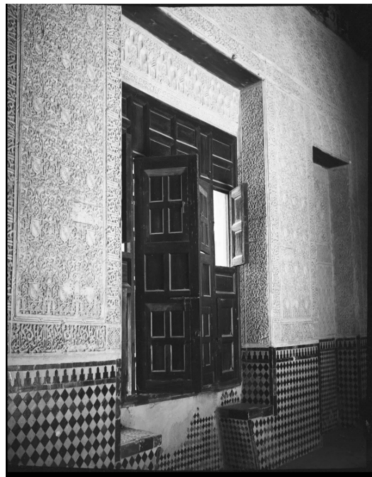
Figure 23. Ceramic dado on the north wall of the Cuarto Dorado, with pieces missing beneath the mullioned window (undated). © Archivo del Patronato de la Alhambra y Generalife, Photograph Collection, F-033020.
