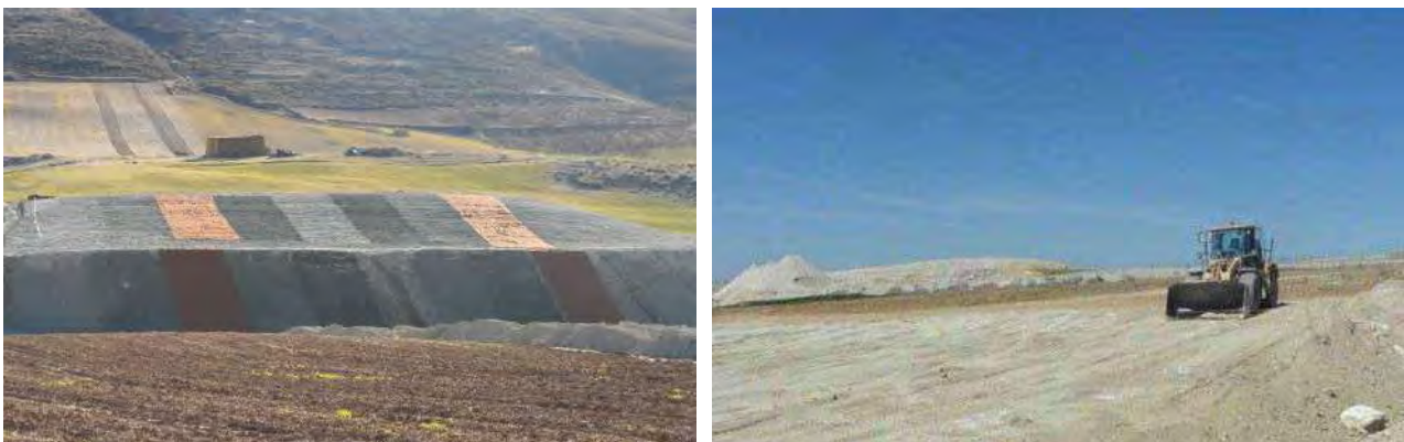
Figure 5. View of the slopes experimental area where different surface treatments can be observed ( left ). Gypsum spoil area conditioned for lichen translocation experiments ( right ).
