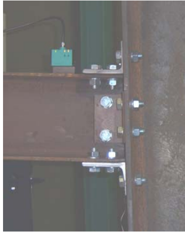
Figure 11. Deformed connection configuration for Test1
