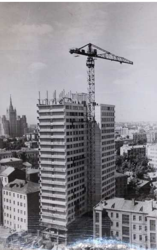
Figure 133. Kalinin Avenue (Novye Arbat Street) General view of one building under construction. 1967
