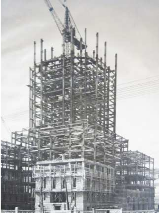
Figure 127. Hotel on Kalanchevskaya Street. General view of construction process. Arc. Polyakov L.M. and Koreckiy A.B. 1951
