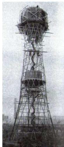
Figure 13. Two-section tower (with two tanks) in Yaroslavl, 1911. Design and the construction process.
