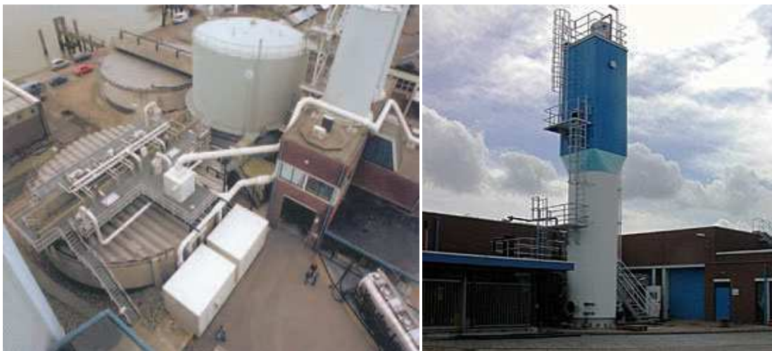
Figure 1. Full-scale partial nitritation (left) and anammox (right) bioreactors in Dokhaven wastewater treatment plant.
