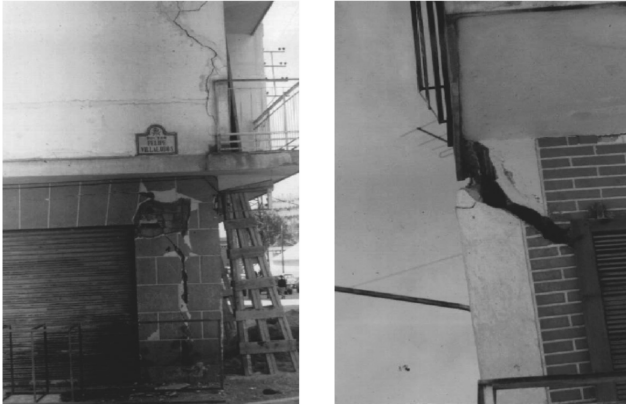
Fig. 14. Deterioration in a building in the Calle Pareja Yébenes, which led to the building being evacuated and demolished.
