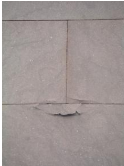
Figure 5-2 Detail of deteriorated Portland Brownstone blocks that belong to the façade of the Victoria Mansion (MA, USA). The damage originates where the vertical mortar joint meets the block below. This could indicate that salts leach from the mortar and initiate damage in the stone (however, it might also mean that water runs down the joint and keeps the stone wet at that location).
