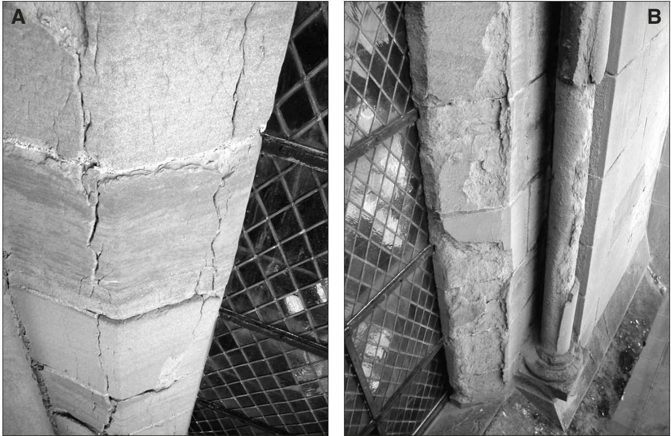
Figure 1. (Upper) Cracks in stone (molasse) on left side of window in Lausanne Cathedral; (Lower) damaged stone on right side of the same window.
