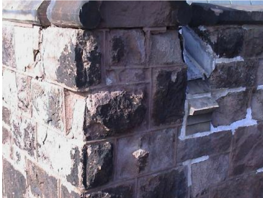
Figure 4-9. Northeast corner of Edwards Hall at Princeton University. The image shows the presence of black crusts in zones exposed to rain where gypsum crusts tend to be washed away. Such crusts in exposed zones are expected to be of biological origin and to contribute to moisture retention, thus increasing freezing damage, Young et al. (1995).
