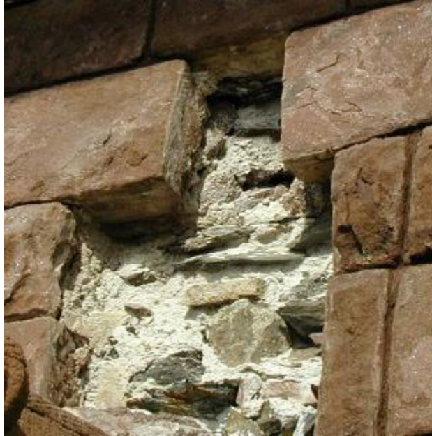
Figure 2-1 Picture of a Portland Brownstone front at St. Mary's showing the masonry wall behind the stone façade (Picture provided by Ivan Myer)
