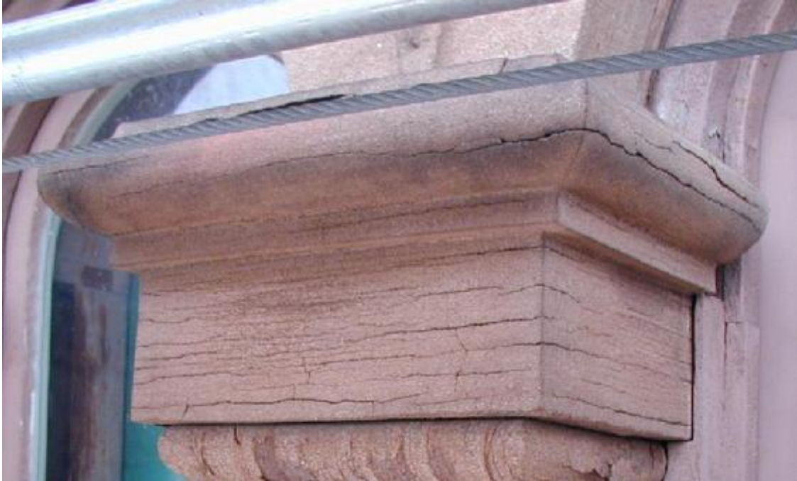
Figure 5-6. Portland Brownstone anisotropy should result in an anisotropic crack spacing, departing from typical mud-cracking pattern. This capital from the Victoria Mansion shows damage consistent with this interpretation (Picture provided by I. Myjer).
