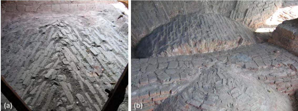
Fig.16. Detail of the construction: (a) Bricks arranged like a fish spine in the transversal vaults, (b) Connection between one of the lateral vault and the wall.
