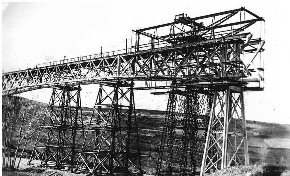
Figure 8. Assembly of the superstructure of the Gor viaduct in 1905. Photograph taken by Gustave Gillman. Courtesy heirs of Gustave Gillman.
