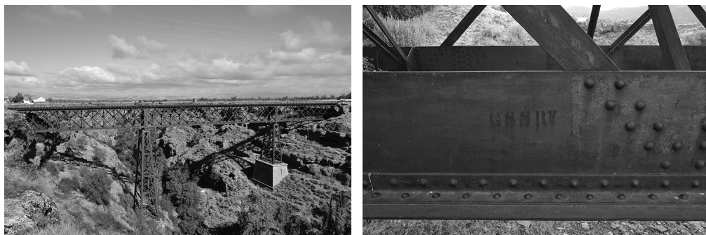
Figure 6: Baúl viaduct as finally built in 1904. Note the 'GSSR' marks on the bottom chord (detail). Photographs by the authors.
