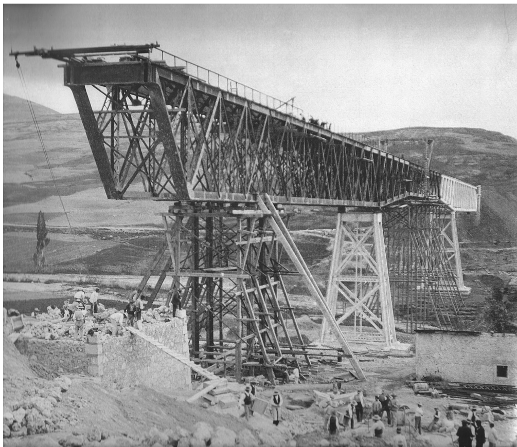
Figure 10. Works to build the new abutment, Winter 1906. Workers are demolishing the old abutment, while the viaduct is provisionally resting on trestles. Photo by Gustave Gillman, 1906. Courtesy heirs of Gustave Gillman.
