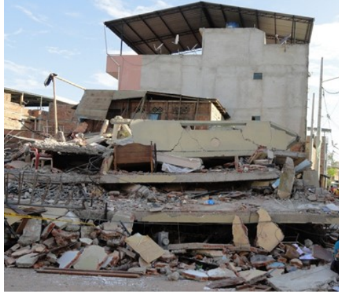
Figure 2: Example of dissimilar behaviour of masonry infilled frame structures after the Pedernales earthquake in Ecuador 16-04-2016 (courtesy of Eng. Raúl Hernández). Note that the building shown at the back of the picture revealed good performance, in contrast to the one at the front.
