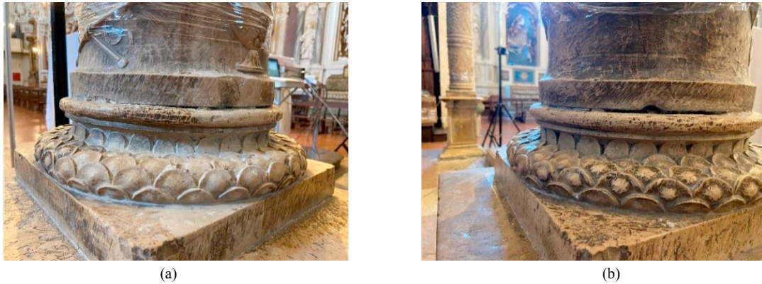
Fig. 2. Images of the state of degradation of the joints observed at the base of the columns.
