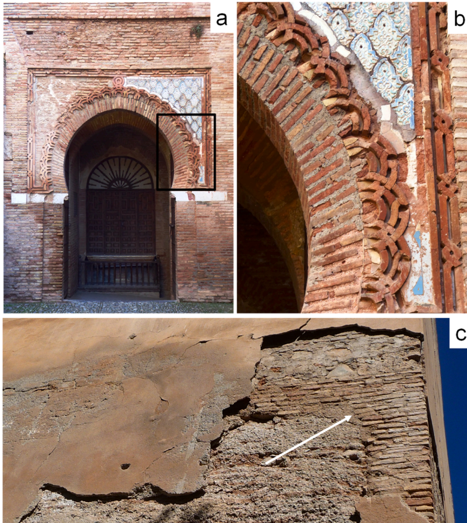
Fig. 1. Bricks of the Alhambra fortress (Granada, Spain). (a) General view of the “Puerta de la Justicia” (Gate of Justice), (b) detail of decorative masonry at the “Puerta de la Justicia” showing some material loss, and (c) historic reconstruction of the “Torre del Agua” (Water Tower, rammed earth structure) using bricks (white arrow).
