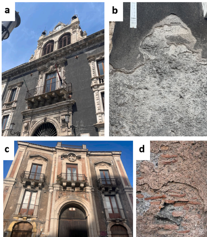
Fig. 1. Examples of use of azolo (a–b) and ghiara (c–d) mortars in buildings of the historical city center of Catania and corresponding degradation forms: a) Palazzo Tezzano, built in the first half of the 18th century, and b) detail of salt efflorescence on the main façade and detachment of the outer layer; c) Esedra in Dante square, built in the second half of the 18th century, and d) detail of disaggregation and detachment of mortar portions from the main façade.
