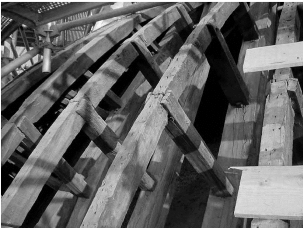
Figure 74 Concepción Real de Calatrava Church. Interior of the structure while restoration works (Estepa, 2015).
