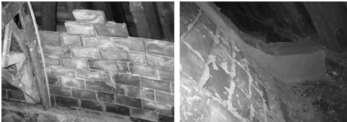
Figure 72 Tile inner dome, with a single layer of brick and with a reinforcement up to one third of the height (Martín, 2009).
