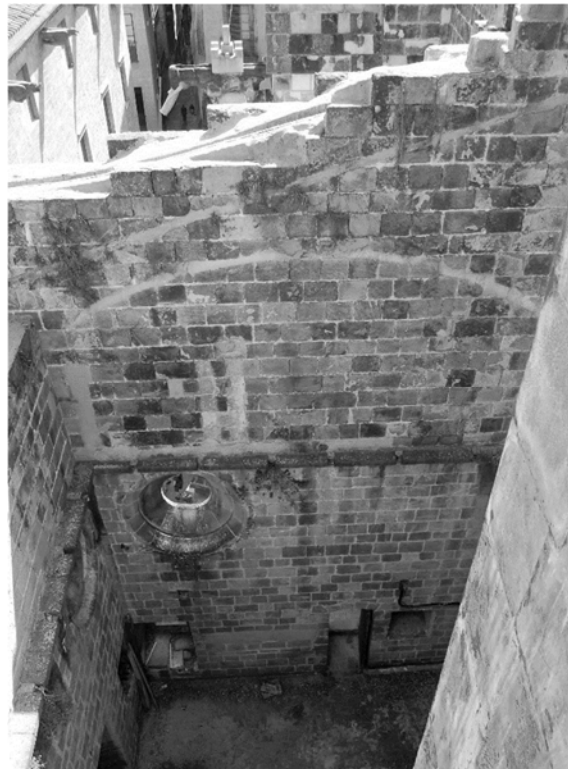
Figure 60 Trace of the tile vault and the roof in the royal chapel of the Cathedral of Barcelona (Conejo da Pena, 2012).
