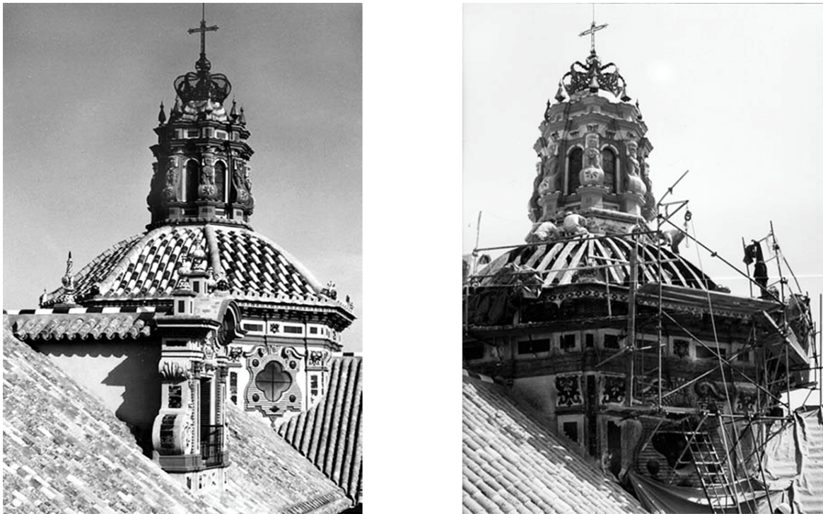
Figure 68 Dome of Iglesia de la Magdalena in the San Pablo Convent in Seville. Repairs works in the years 1989-1991 (Pinto, 2005).
