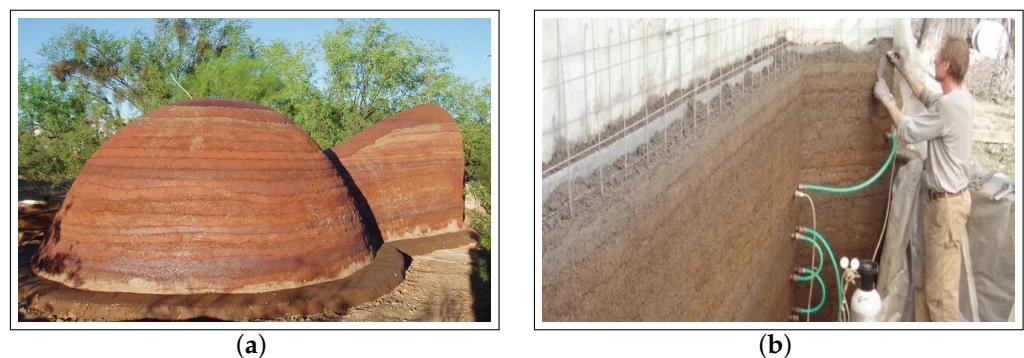
Figure 3. Ferrock construction examples. (a) Dome structure made of ferrock in USA. Picture taken from https://www.certifiedenergy.com (accessed on 15 October 2023). (b) The process of building a ferrock wall. Picture taken from https://www.pbs.org (accessed on 15 October 2023).
