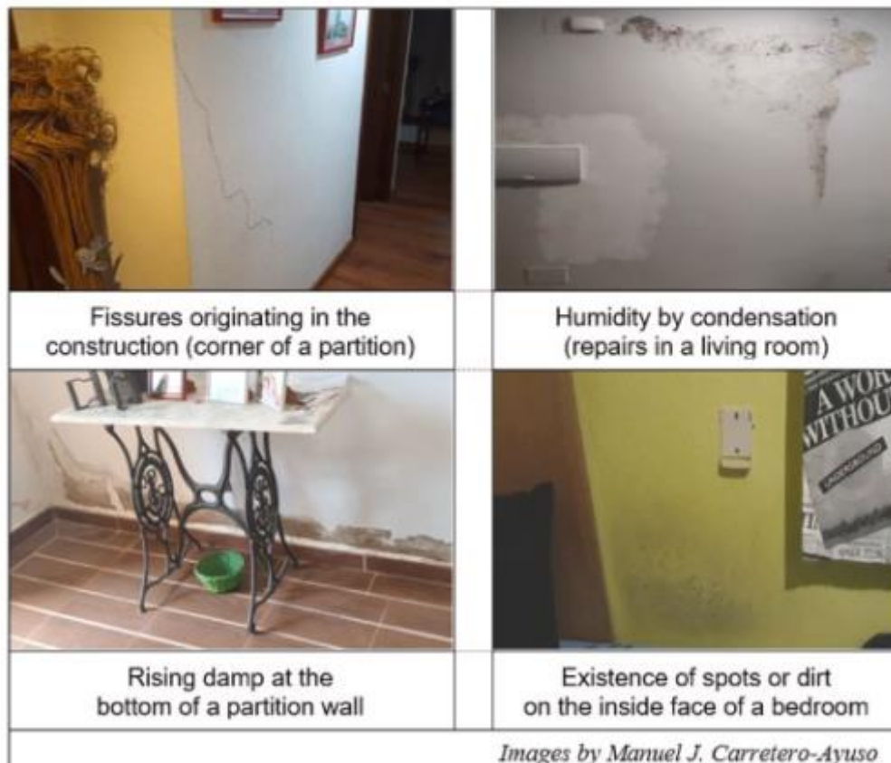
Fig. 12. Photographic examples of some damages in partition walls.
