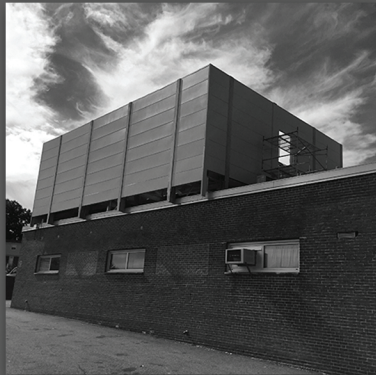
ROOFTOP NOISE BARRIER WALL SYSTEM
