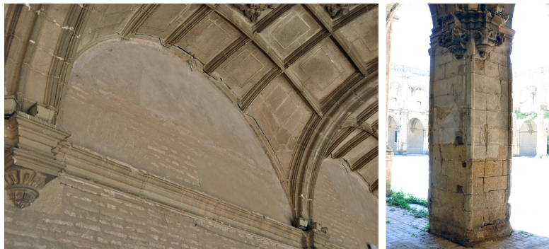
Fig. 5: Detected damage in the main cloister of the Monastery of San Jerónimo.
