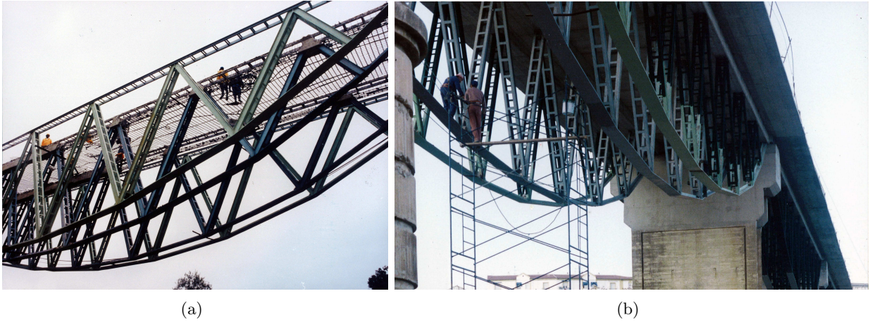
Figure 7: Views of (a) initial and (b) final operations of deck's width increment (1992).
