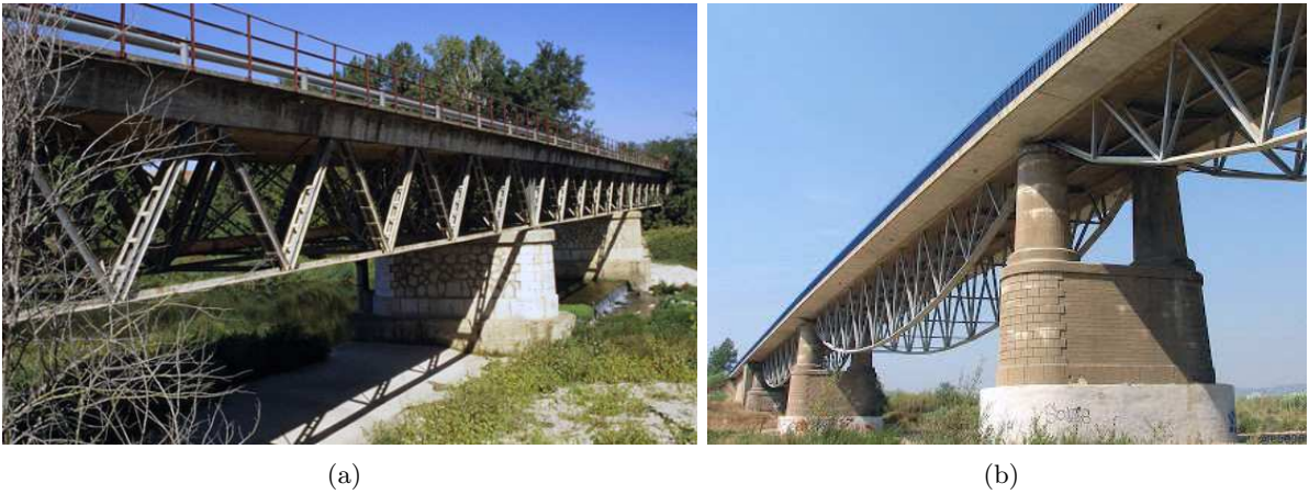
Figure 2: Views of (a) Muga Bridge, 1939 (Girona, Spain), and (b) Tordera Bridge, 1939 (Barcelona, Spain).
