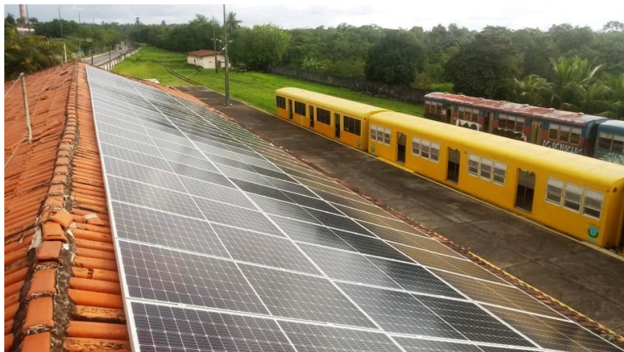
Fig. 2. Photovoltaic systems from Joao Pessoa office during (top) and after (down) installation.
