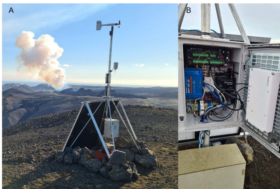
Fig. 3 (A) Example webcam installation operated by Civil Protection. Power is supplied by two 200 Ah, 12V batteries charged by a solar panel, which also powers a small weather station. (B) A weather proof box contains the 4G GSM modem and power management
