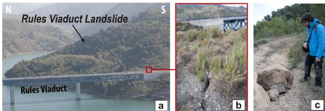
Figure 9. (a) Photograph of the Rules Viaduct Landslide. (b) Opened cracks near the southern abutment of the Rules Viaduct. (c) Sinkhole within the anthropic filling.
