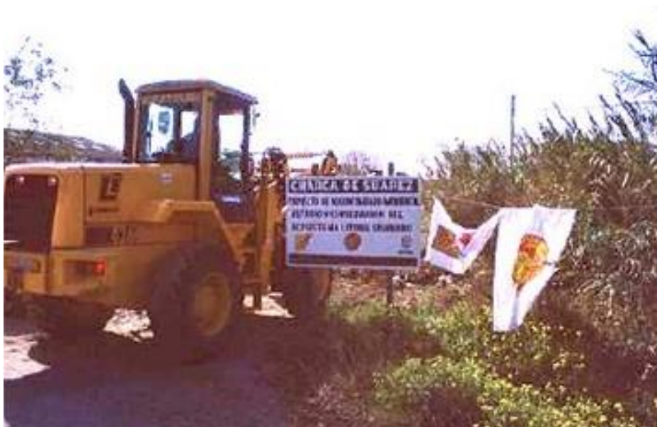
Figure 1.3.- Wetlands dewatering project stopped by workers of LCS reserve and the inhabitants of Motril.
