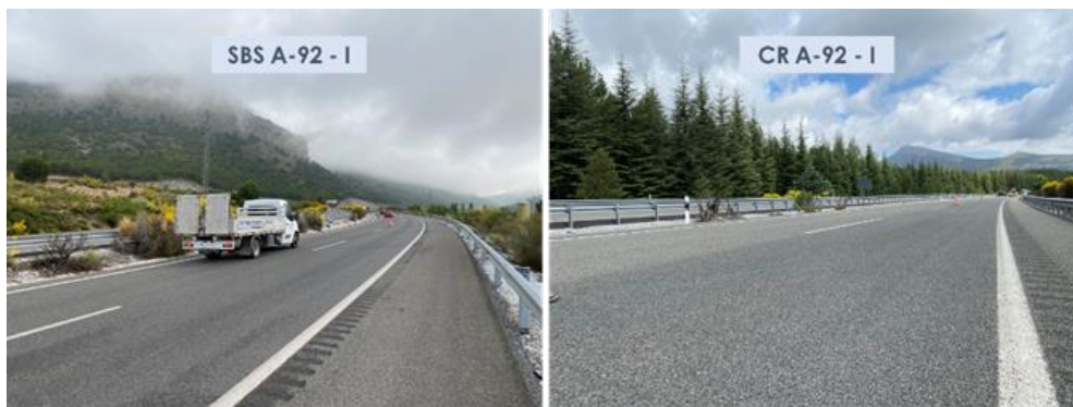
Figure 4.2.4. Aspects of the surface asphalt layers manufactured with SBS and crumb-rubber-modified binders on A-92 highway after 46 months of service life.
