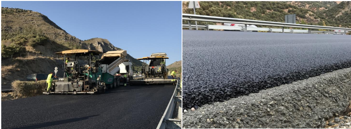
Figure 4.3.13. Images from the spreading and compaction of the CRMB-WMA with a thickness of 3 cm.
