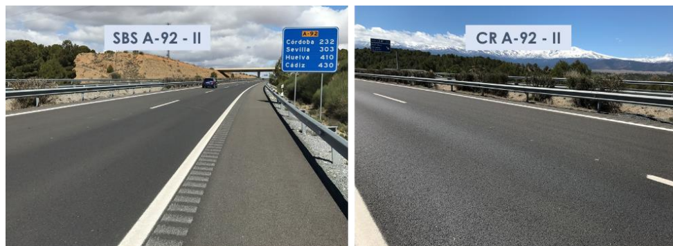
Figure 4.2.5. Aspects of the surface asphalt layers manufactured with SBS and crumb-rubber-modified binders on A-92 highway after 36 months of service life.
