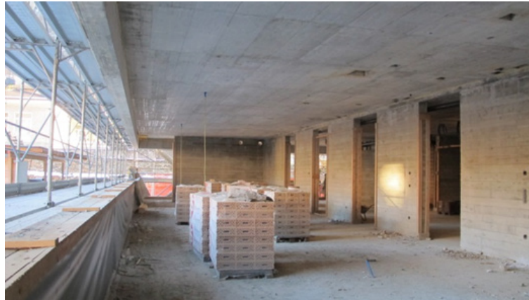
Figure 1.56. The “Elena Cerio” retirement home in Giornico – Cantilevered room block resting on the walls on the ground floor (photo by Pedrazzini Guidotti sagl, Lugano)
