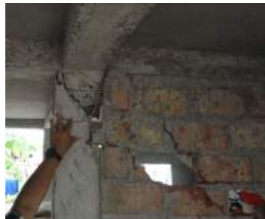
(b) Short column effect due to masonry infilled corner compressive crushing.
