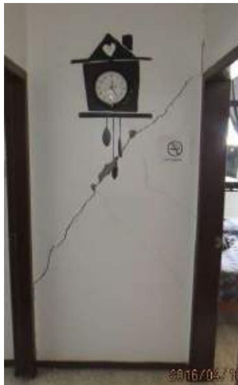
Figure 1.2: Broken wall of the sixth floor department from an eight story building, located in the center of Guayaquil city, after the seismic event of 2016.
