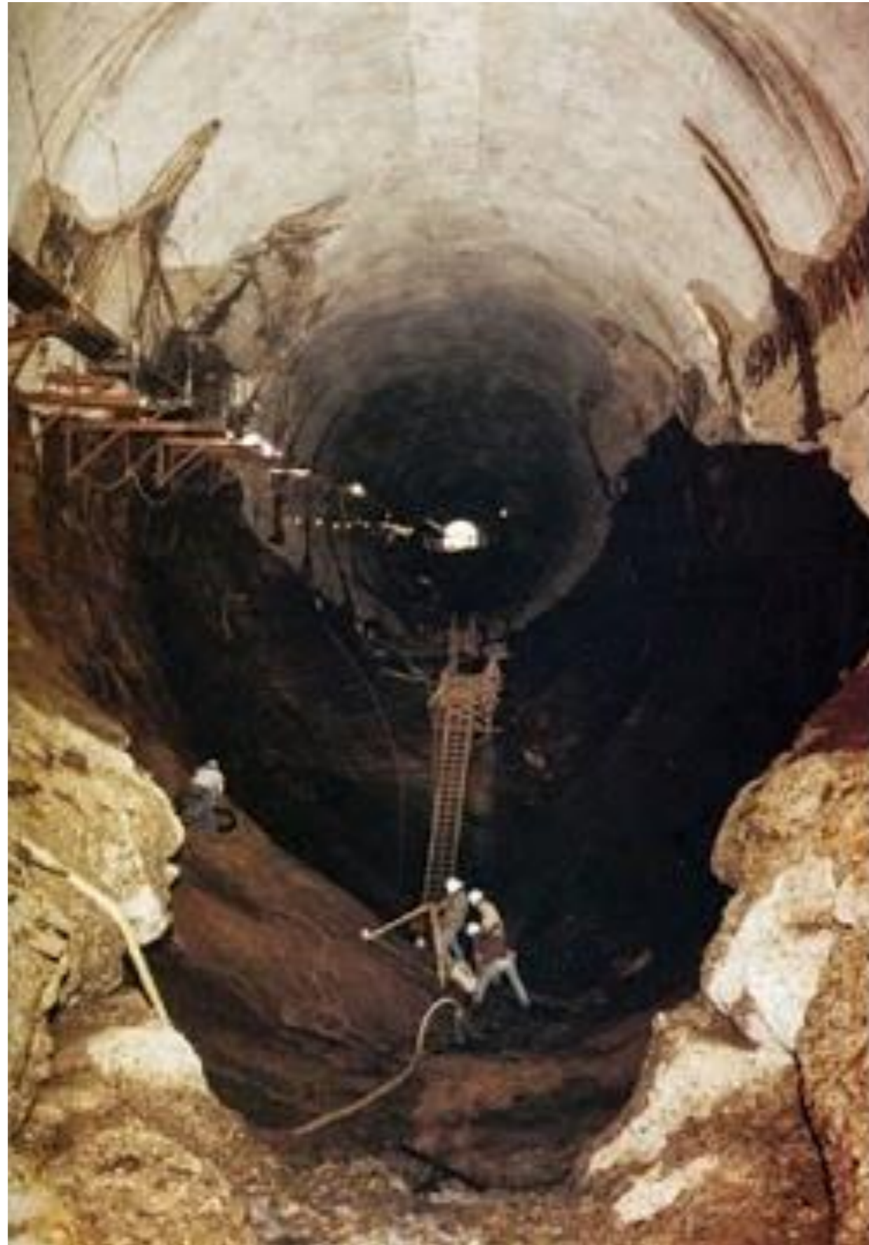
0.91 m-thick concrete tunnel spillway Cavitation damage during the 1983-84 flooding
