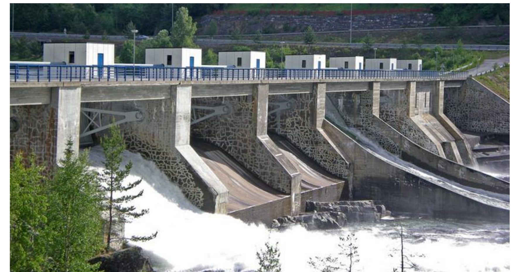
ASR-induced map-cracking on a dam in Norway.
