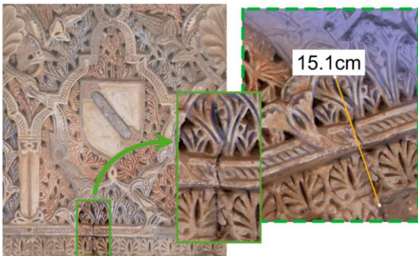
Figure 7: Information on fissures and cracks identified in the photogrammetric model.
