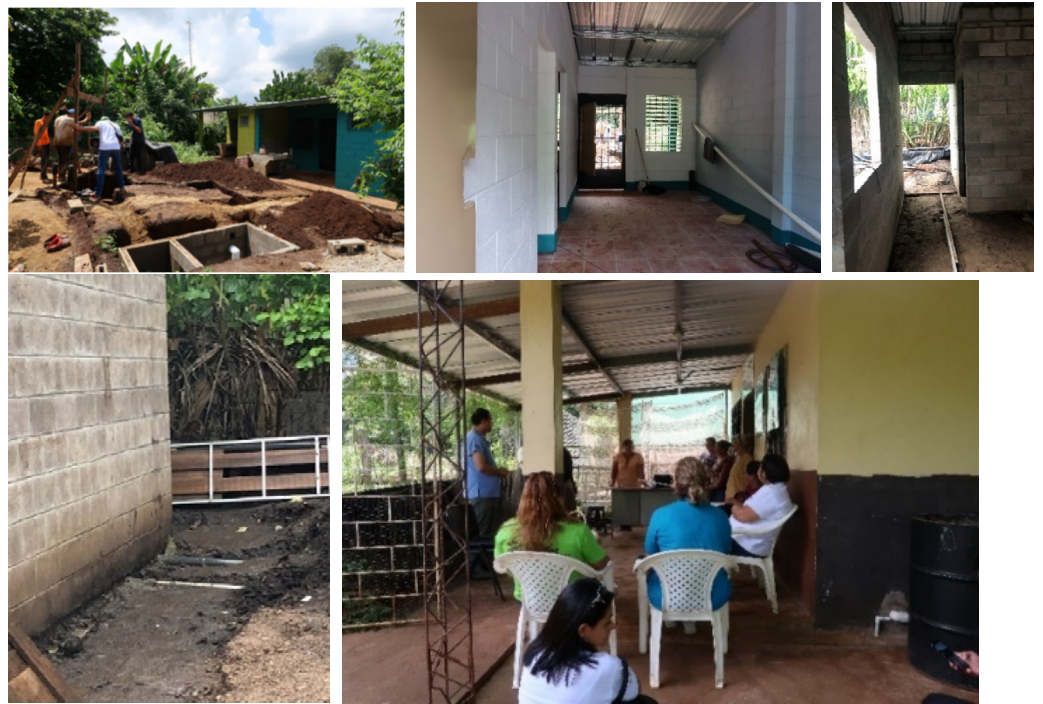
Figure 4. Visits to the works in progress of extension and improvement of the houses.
