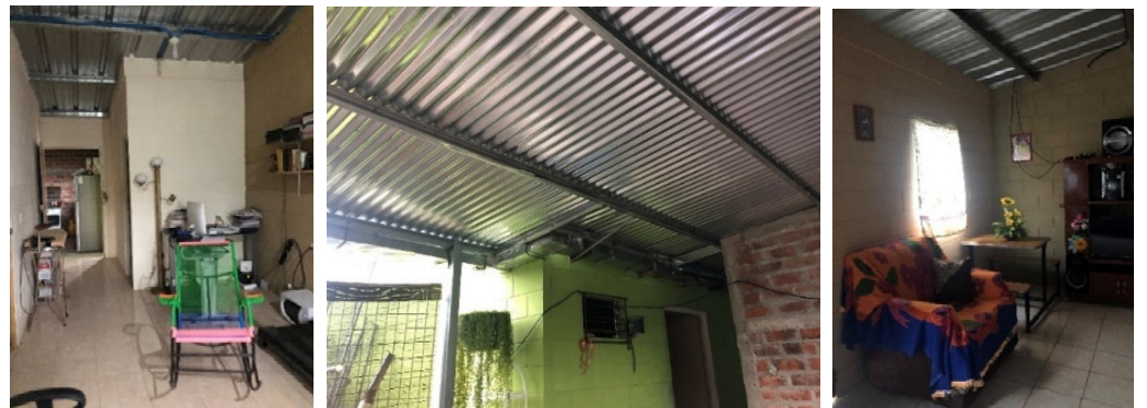
Figure 2. Visit to the interior of the Habitat NGO pilot homes.
