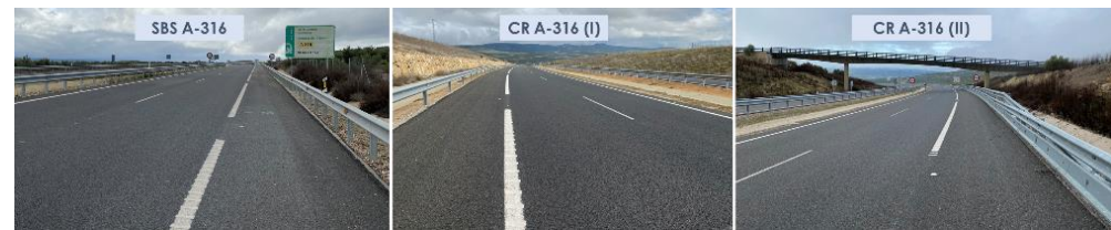
Figure 3. Aspects of the surface asphalt layers manufactured with SBS and crumb-rubber-modified binders on A-316 highway after 63 months of service life.
