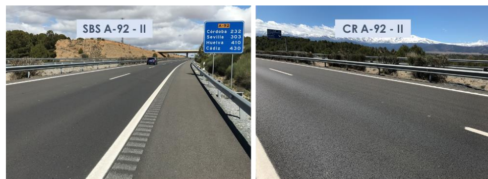
Figure 5. Aspects of the surface asphalt layers manufactured with SBS and crumb-rubber-modified binders on A-92 highway after 36 months of service life.
