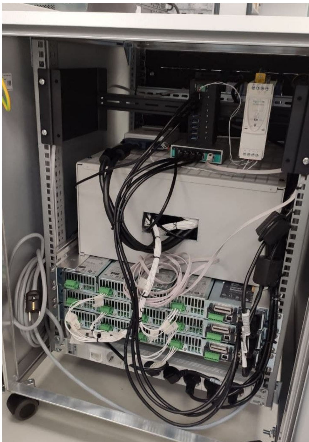
Figure 5.11 – Rack back view
