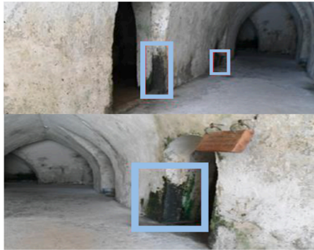
Fig. 7. Deterioration of the plaster, green spots on the wall of the vault, and rising damp on the floor.
