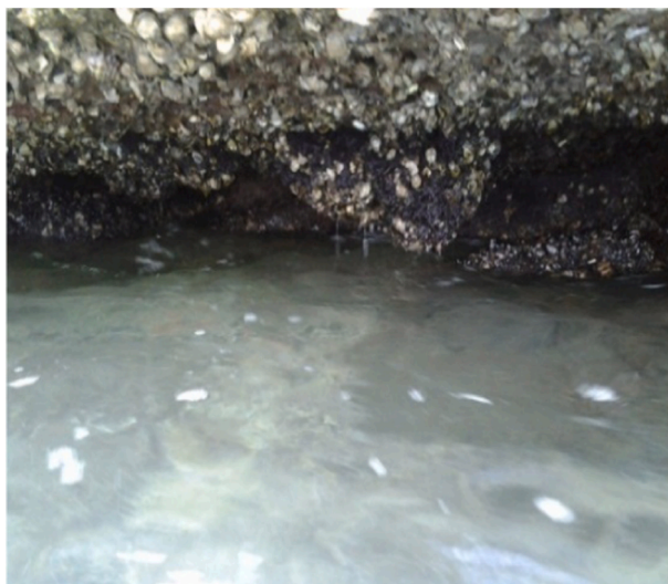
Fig. 9. Scour and deterioration of the stone material in the external part of the bathroom.
