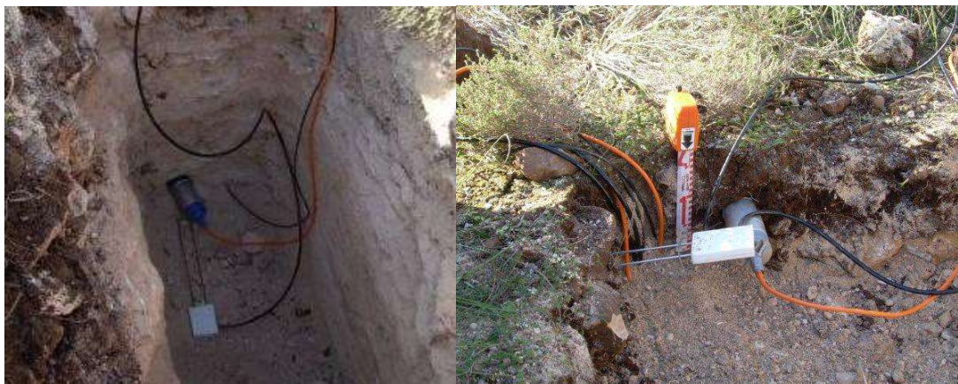
Figure 12. CO 2 , temperature and soil water content sensors at 1.50 m (left) and 0.15 m (right) before refill the boreholes during deep profile installation. Photos from in Balsa Blanca experimental site.
