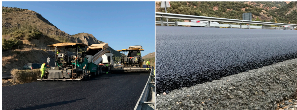
Figure 13. Images from the spreading and compaction of the CRMB-WMA with a thickness of 3 cm.
