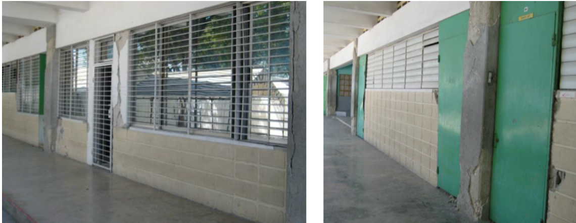
Figure 6.8: Frames in D1. Windows in one span and openings in the other span (photo Chungwook Sim et al).
