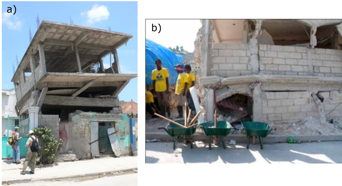
Figure 6.1: a) Irregularities in the vertical dimension triggers soft story effect (photo Chungwook Sim et al.). b) Captive columns. Short-column effect. (photo Rebekah Green. EERI Special Earthquake Report-May 2010).
