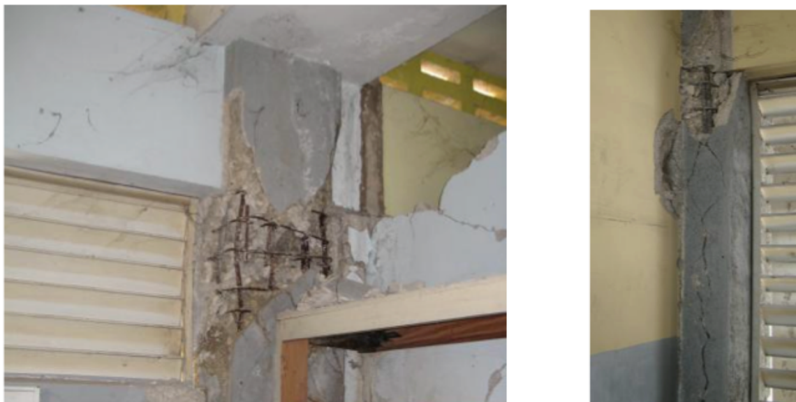
Figure 6.9: Buckling of rebars. Shear crack on the longitudinal axis of the column.
