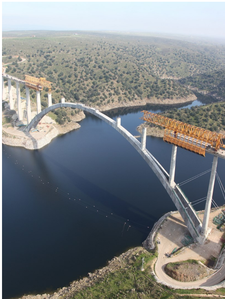
Figure 4.1: The viaduct over the Almonte river in construction phase. Source: FCC Construcción, S.A. official website ( http://www.ciudadfcc.com/ ).
