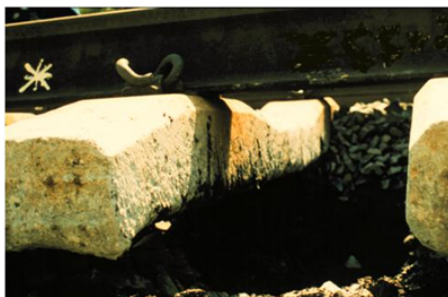
Figure 24. Slurry abraded concrete ties.
