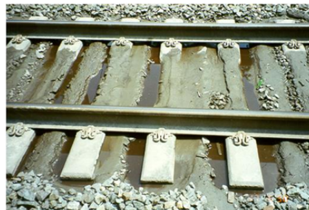
Figure 23. Slurry (mud) filled ballast.
