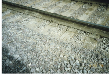
Figure 22. Fouled ballast due to subgrade attrition and pumping of fine material.
