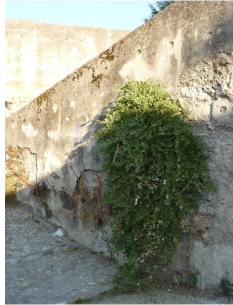
Figure 1-21. Plant growth and damage due to capillary rise, Albayzin, Granada, Spain.
