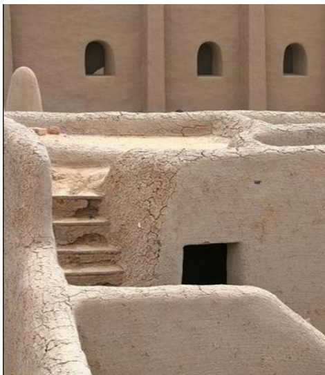
Figure 1-18. Drying cracks in an earthen structure in Djenné, Mali (www.flickr.com).
