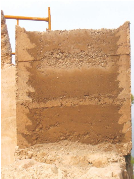
Figure 1-13. “Tapia calicostrada” Castell Vell de Castellón de la Plana, Spain (Font and Hidalgo 2011).
