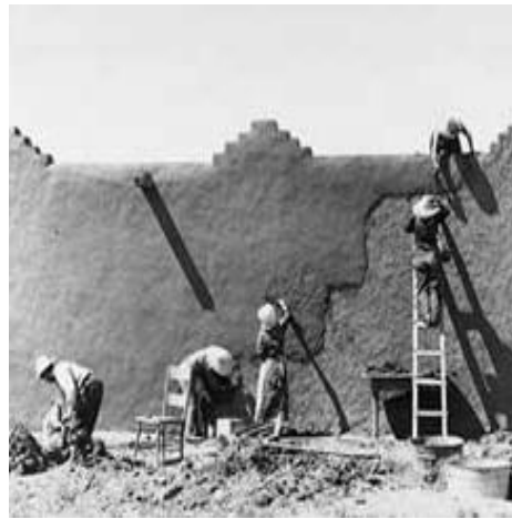
Figure 1-11. Renewal of the surface coating of an adobe wall in Chamisal, New Mexico ( www.en.wikipedia.org ).
