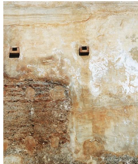
Figure 1-19. Salt efflorescence caused by Portland cement used in a conservation intervention (Castillo de Santa Catalina, Granada, Spain).
