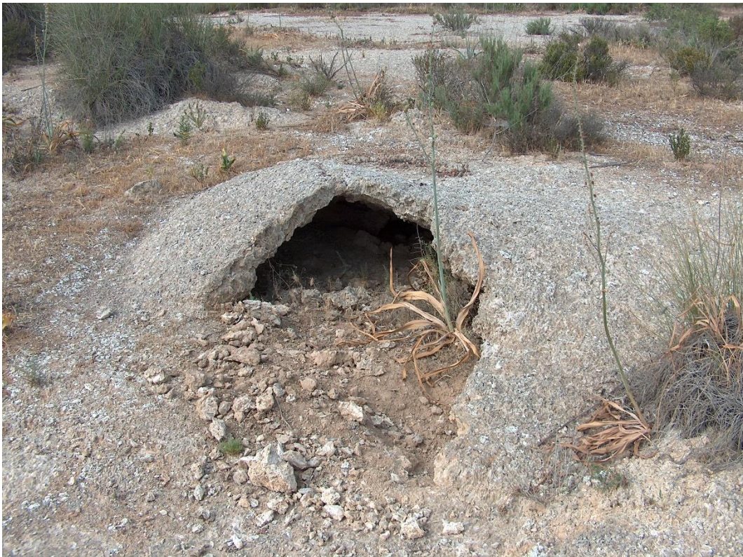
Photograph 64.- Partially-collapsed, igloo-like gypsum structures. These structures are presumably linked to quick de-compaction, and occur on top of the gypsum outcrops (Sorbas Basin. Marchalico-Viñicas).
