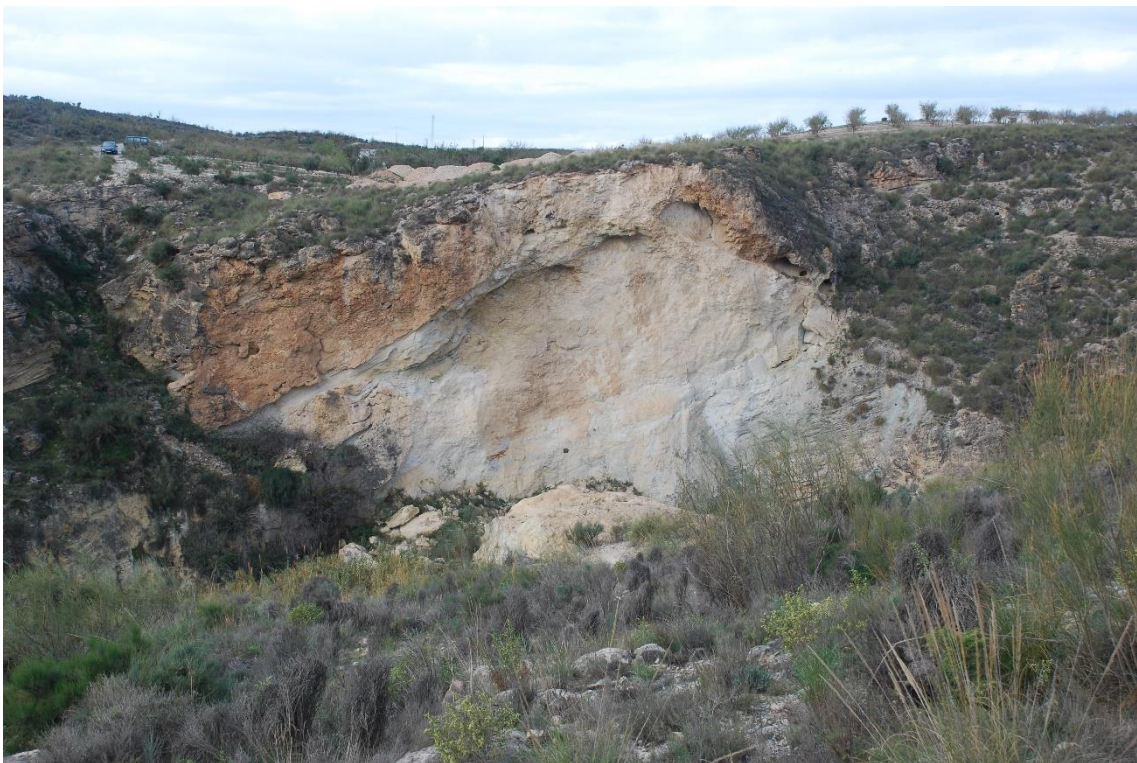
Photograph 75.- Part of wall seen in the previous picture, consisting mostly of sands, has collapsed very recently (Cuenca de Sorbas. Rambla de Góchar).
