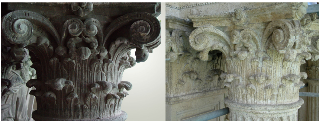
Figure 4. Black crust development on the carbonate stone surface of one decorated column of the Cathedral of Granada ( Portada del Perdón ) due to atmospheric pollution (left). The same column after the cleaning process (right).
