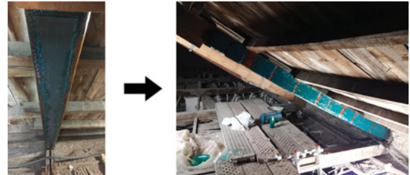
Figure 19. Rehabilitation process of the rafter. Left-hand side: placement of the CFRP lamella. Right-hand side: final state of the reinforced element. Image by authors.
