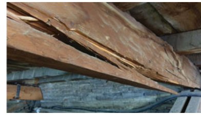
Figure 18. Damaged rafter before the repair process. Image by authors.
