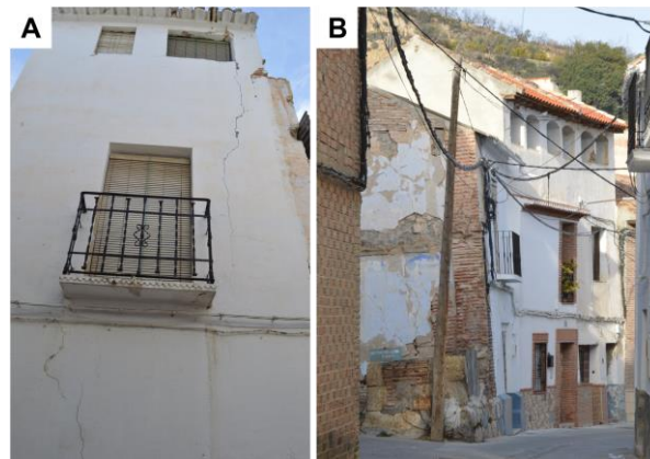
Figure 4. Buildings of the Albuñuelas village affected by slight deformations (A) and tilting (B) due to the activity of a deep-seated landslide on which the village is located.
