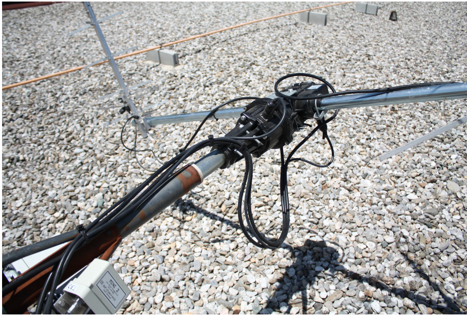
Figure 4.10 – Rotor mounted on the mast
