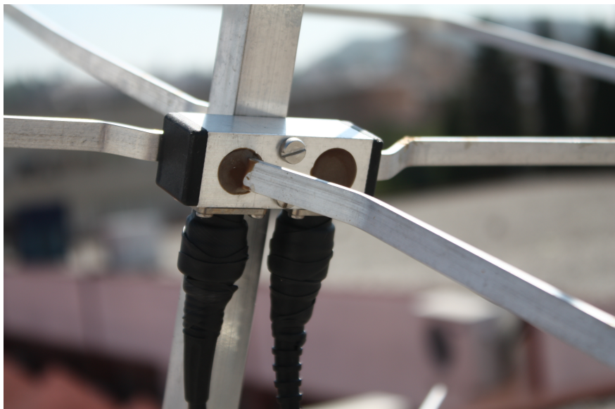
Figure 6.7 – Self-amalgamating tape covering the two connectors of the 70 cm antenna
