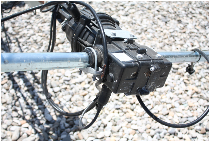
Figure 6.19 – Ripped cable on the side of the rotor
