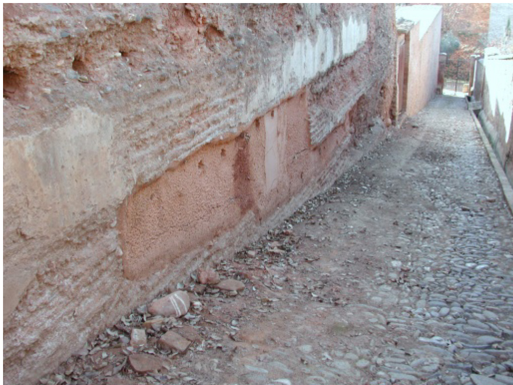
FIGURE 6. Restoration of a rammed earth wall with significant loss of mass at the base.
