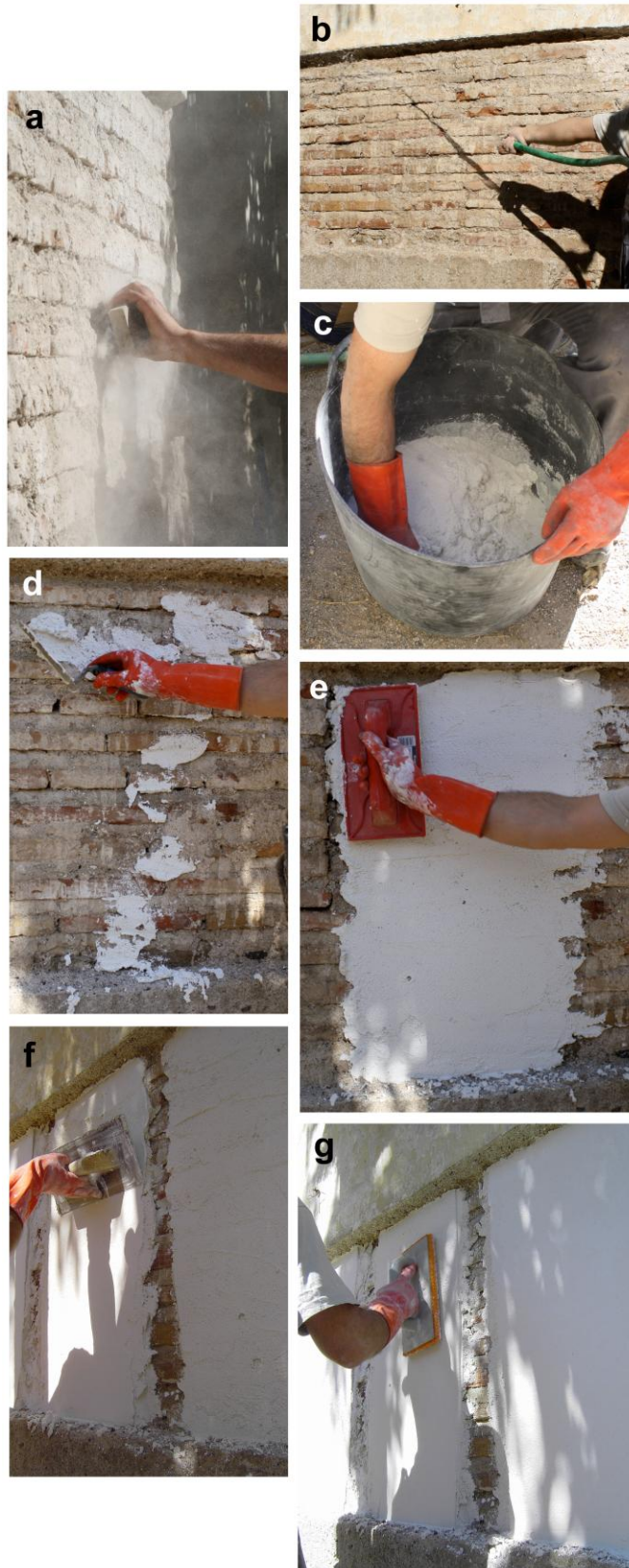
Figure 1 Steps of the application of the rendering mortars in the Vargas Palace (Granada): brushing (a) and wetting (b) of the wall surface; mortar mixing (c); application of the mortar (d); spreading of the first layer (e); application and spreading of the second layer (f); trowelling of the surface (g).
