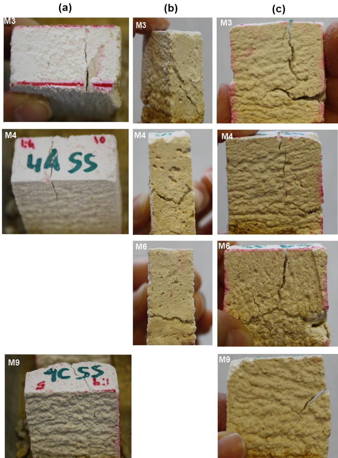
Figure IV.2.4 Images of the different deterioration forms appeared in the mortars samples submitted to the WS+SS test (weathering study and salt resistance by capillary absorption): (a) Fissures developed after 4 cycles in samples M3, M4 and M9. (b) Efflorescences appeared after 6 cycles on the side surfaces of samples M3, M4 and M6; spalling also appears on sample M9. (c) Fractures in form of cross developed in all samples after 6 cycles.
