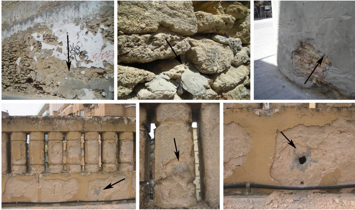
Figure 5 Examples of bad restorations, in which Portland cement (indicated by the arrows) has been used.
